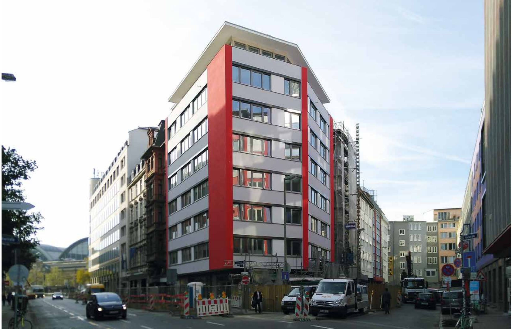
The "NiKa" building during remodelling work. Architecture: Meides & Schoop Architekten. Photo: Ulrich Herding for the "NiKa" project
