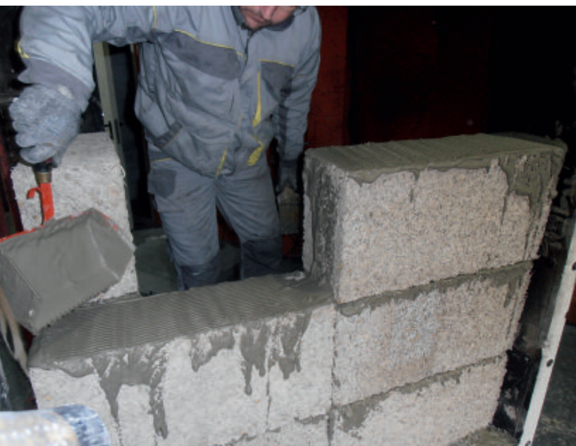
Sustainable building with bio-based building materials (project Grow2Build)
