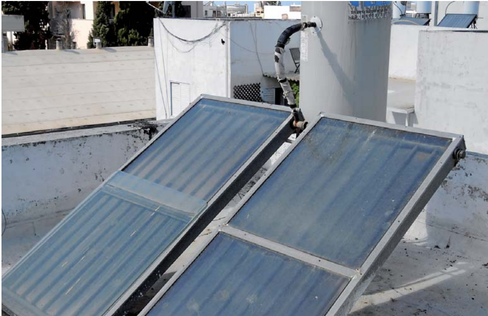
Figure 58: Thermo-siphon installation in Tel Aviv (2013)
