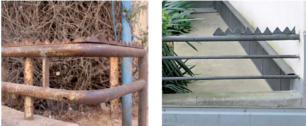
Figure 99: Detail views of steel enclosure elements for building grounds: at left, front yard at Idelson Street 14 in Tel Aviv, (2013); at right, front yard at Nürnberger Str. 3/Danzigerstraße in Karlsruhe Dammerstock (2014). Both enclosures have the same type of serrated upper element.
