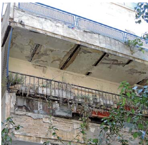
Figure 87: Balcony reinforcement corrosion (Tel Aviv 2013)
