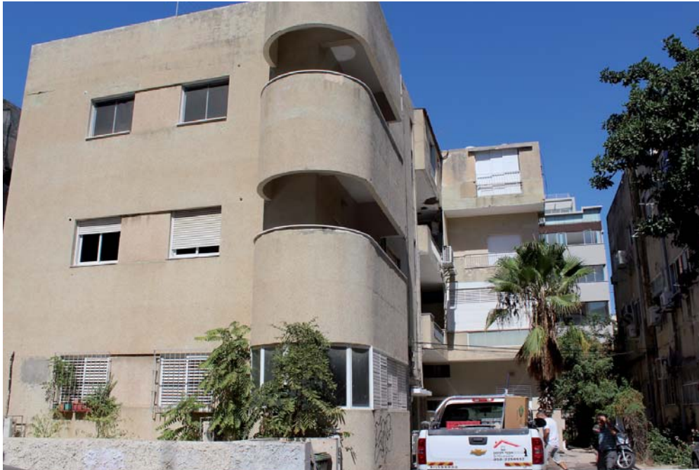
Figure 94: An apartment house being renovated while occupied (balcony enclosures being removed); MazeH Street 31 in Tel Aviv (2013). (The owner is considering installing an elevator.)
