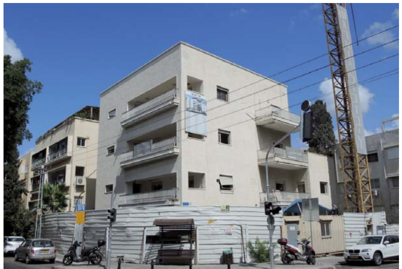
Figure 91: Status of ongoing renovation at Sderot Hen Street 38 in Tel Aviv, in October 2013
