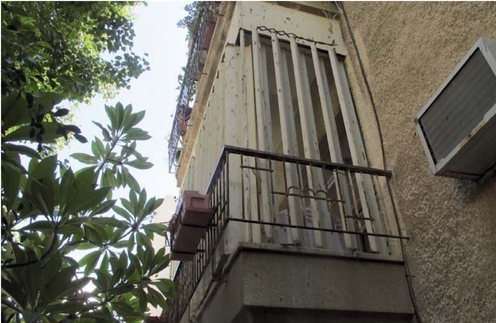
Figure 67: Apartment building (presumably from the 1940s) with characteristic plasterwork, and balcony slats; Gordon Street, Tel Aviv (2013)
