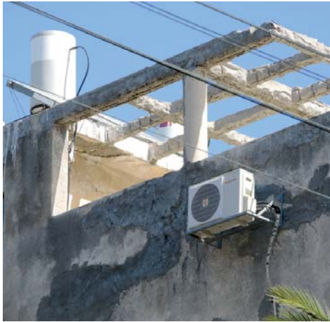
Figure 85: Pergola reinforcement corrosion (Tel Aviv 2013)
