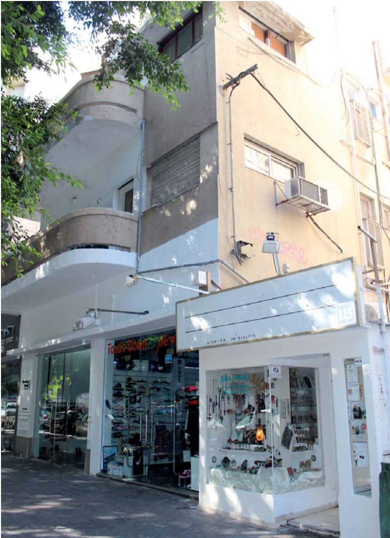
Figure 69: Beige plasterwork that has been partly painted over in white, Dizengoff Street, Tel Aviv (2013)
