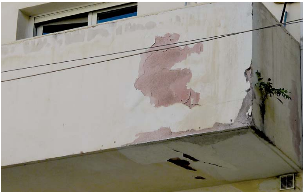
Figure 68: Here, the original reddish brown plaster is visible in places where the paint is flaking off; environs of Bellinson Street and Frug Street, Tel Aviv (2013)
