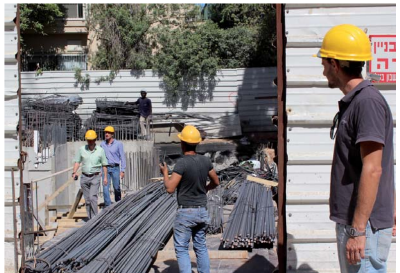
Figure 95: A construction site being operated in an exemplary manner. The extensive measures being carried out will nonetheless result in the loss of substantial portions of the building’s structural fabric and of outdoor appurtenances (Sderot Hen Street 38 [Tel Aviv, 2013])
