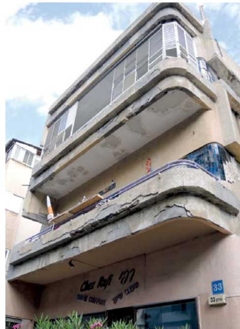
Figure 18: Typical view of a building from the street (2013). This building's balconies are rarely used as such, as many of them were enclosed after the building was constructed (Tel Aviv, 2013)
