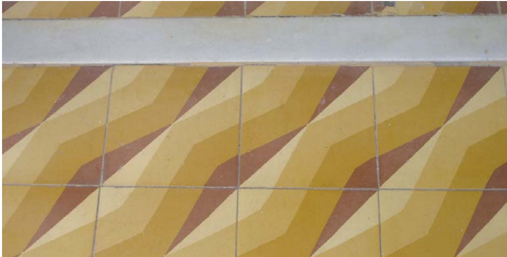
Figure 75: Terrazzo flooring in the living room of a fourth floor apartment at Mazeh Street 31 in Tel Aviv (2013)
