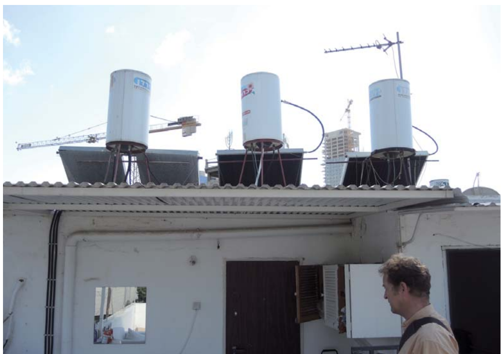
Figure 57: Thermo-siphon installation on the roof of a Tel Aviv apartment building (2013)
