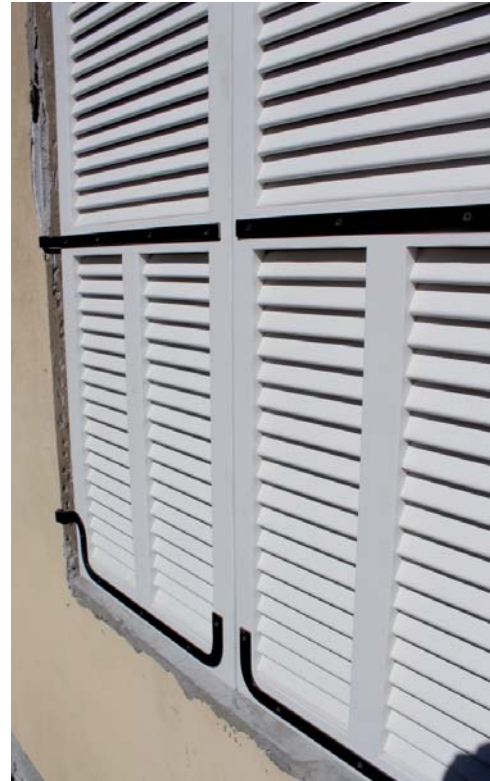
Figure 78: Newly installed shutters in a heritage building (from around 1920) under renovation; Derech Jaffa Street 13, Tel Aviv (2013)
