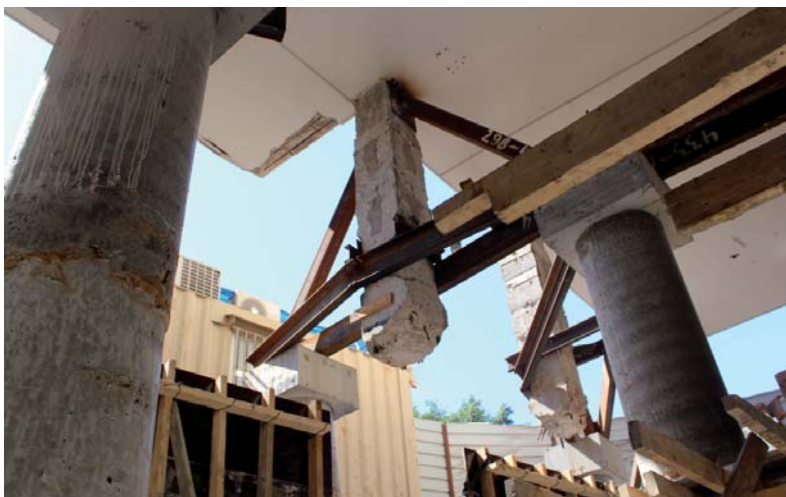
Figure 97: Supported pilotis 85 (pier) under construction between new pillars (view from the new basement) at Sderot Hen Street 38 in Tel Aviv (2013)
