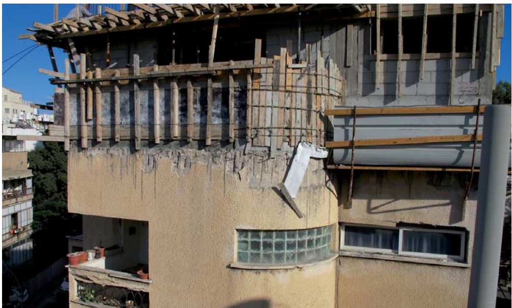
Figure 9: An apartment building to which floors are being added; Aharonovitch Street, Tel Aviv (2013)
