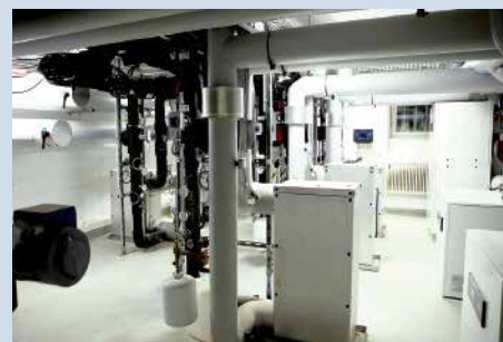
Figure 25: View into the plant room Photograph: Neutraubling Upper Secondary School
