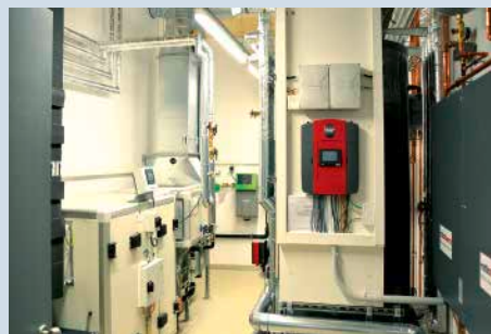
Figure 71: The plant room Photograph: Haase & Bey Architekten
