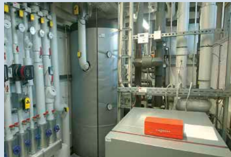
Figure 59: The building services control room Photograph: City of Feuchtwangen
