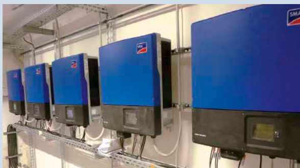
Figure 93: Electrical inverter with power display Photograph: Fraunhofer IBP
