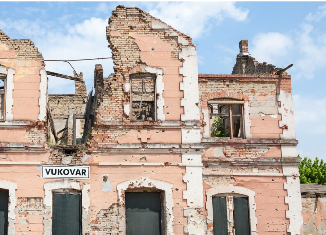
Fig. 17: Vukovar railway station, badly damaged during the battle of 1991. Vukovar, Croatia (iStock.com/BalkansCat)
