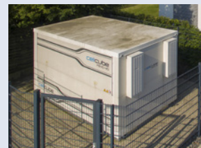
Central electricity storage
