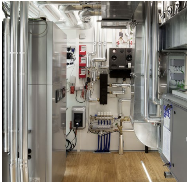
View of the utilities room
