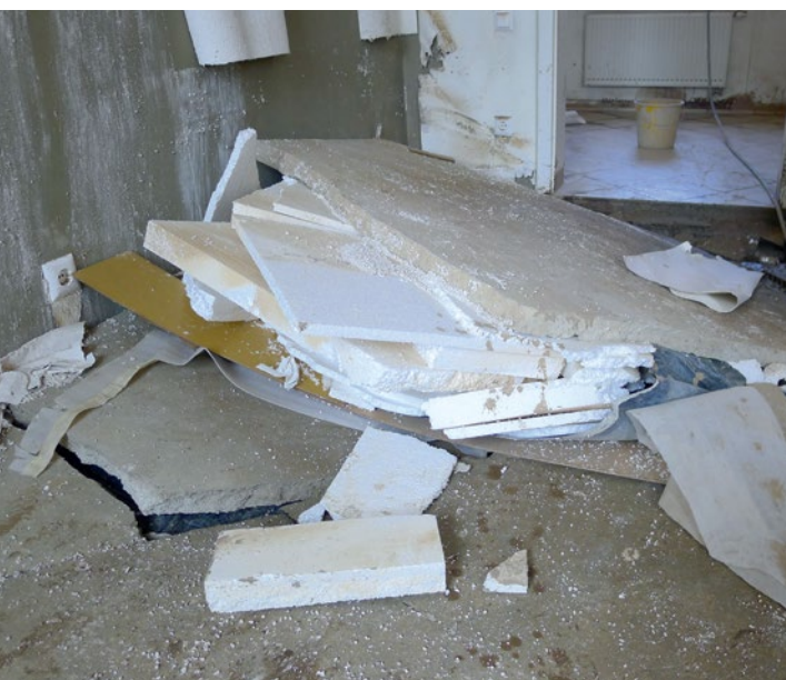
Flood-caused detachment, via floating, of cement screed laid in the “floating” manner
