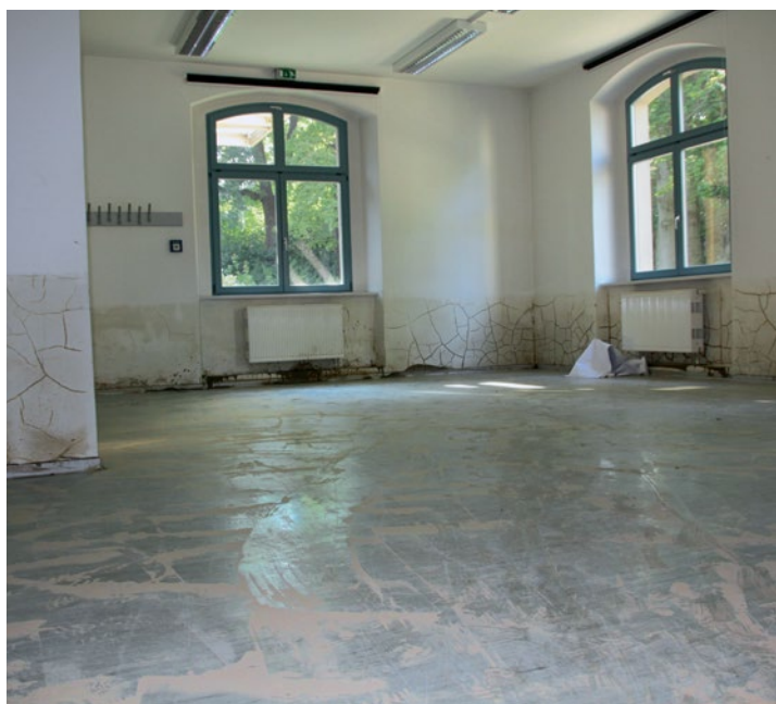
Soaked exterior wall, following a flood
