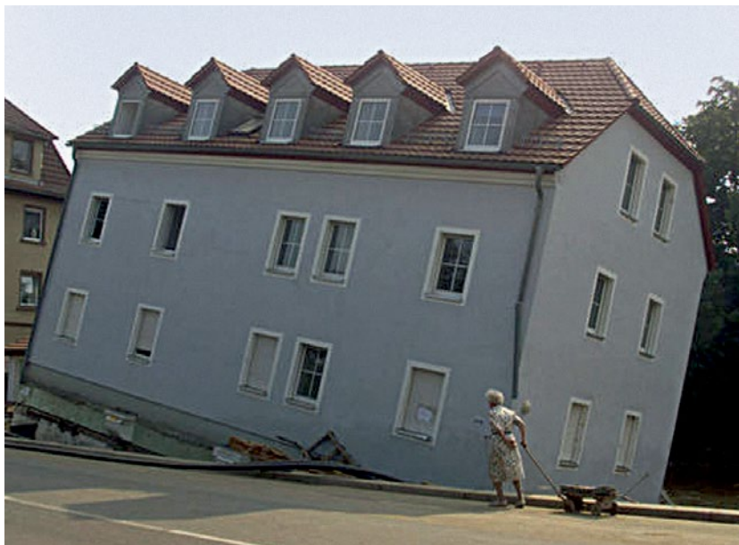
Undermined house along the Weißeritz river
