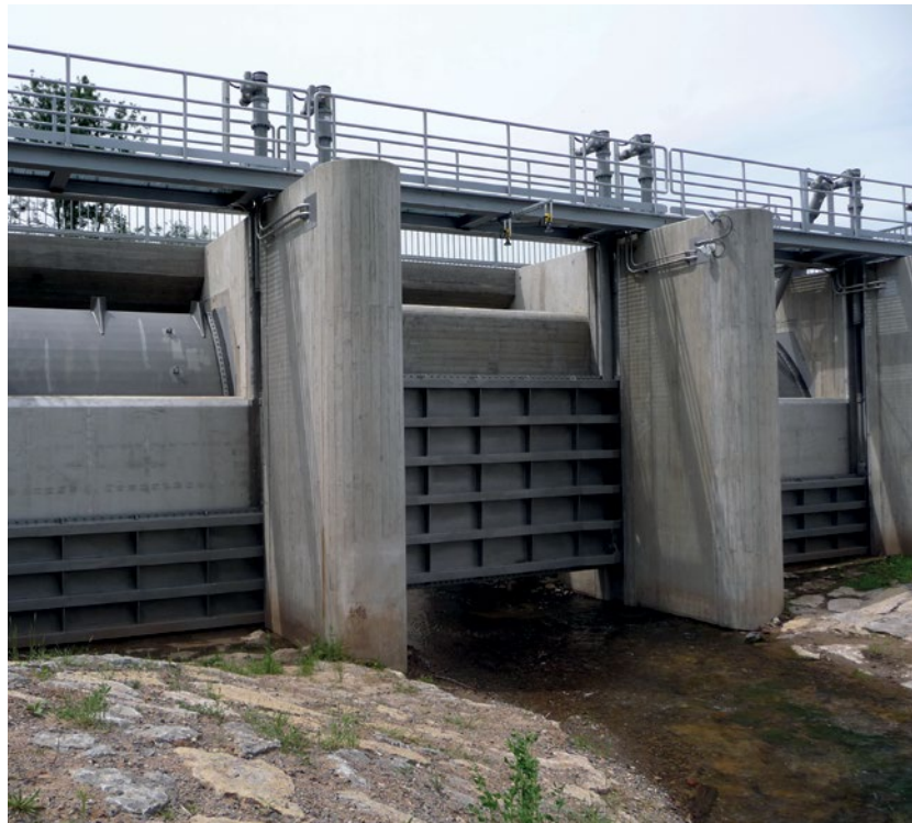
Closing structure for a flood retention basin
