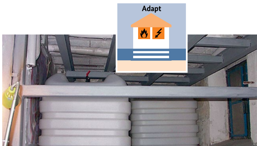
Adapt: for example, by securing tank systems
