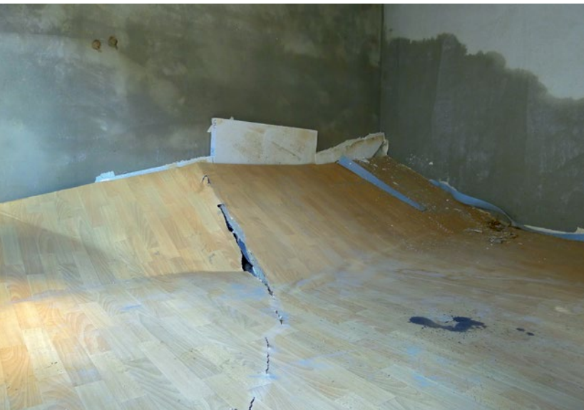
Buoyancy-caused detachment of a floor construction
