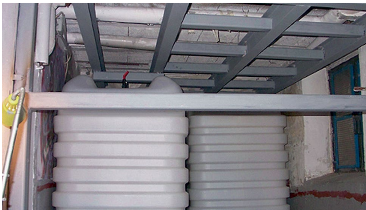
Heating-oil tanks with buoyancy safeguards
