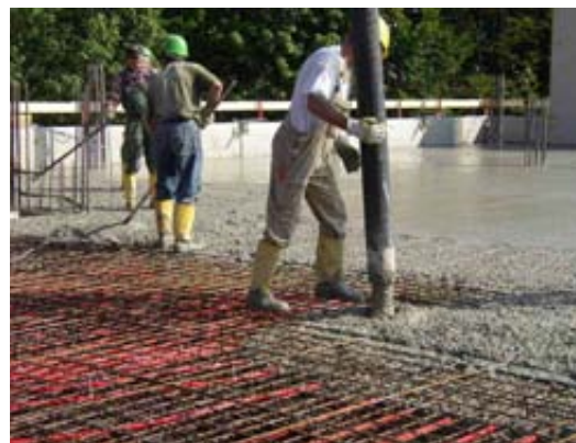
Cementing an intermediate floor with pipelines (red) for building component activation, Photo: Hochschule Offenburg
